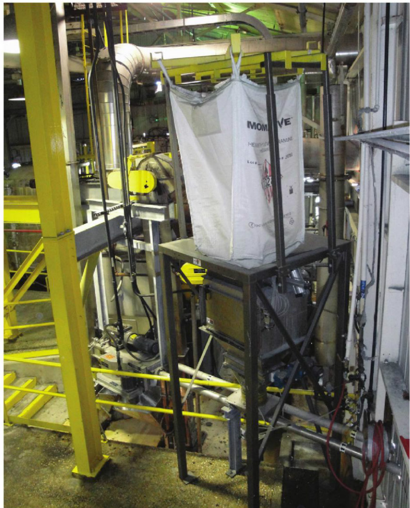
The bulk bag unloader allows for the safe and accurate release of hexamine into the conveying system.
